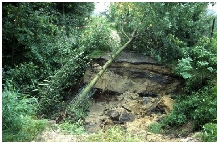
Photo No. 30.: Broken dam of a sewage plant.
