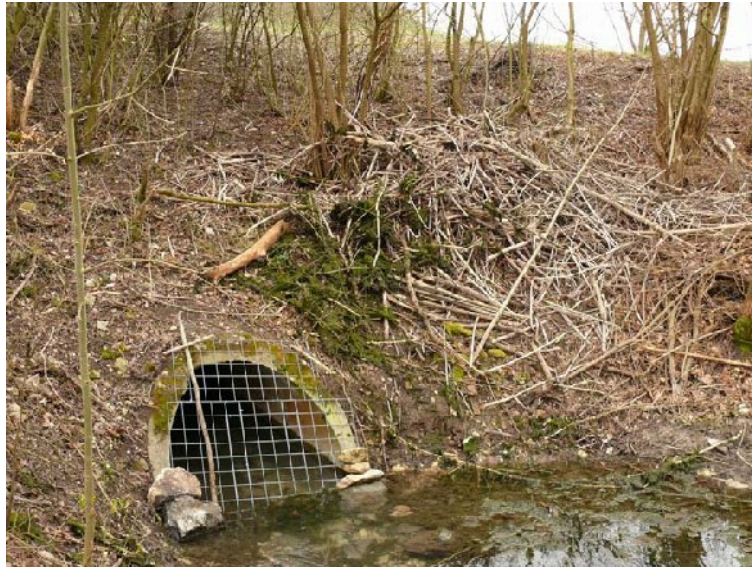
Photo No. 44.: Protection of a culvert with wire grating. On the right the material, that had to be removed from the culvert before blocking
