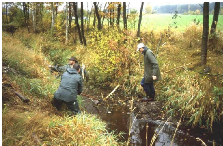
Photo No. 40.: Smaller beaver dams can often be taken out easier and faster by hand than with a digger.
