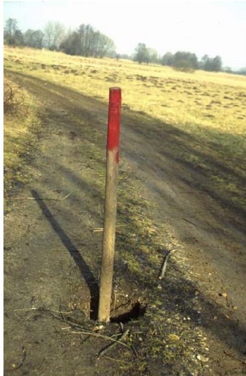
Photo No. 31.: Beaver tunnel under an unpaved access road to fields.
