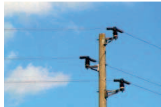
The pole with mounted protectors (Photo from the presentation „Experiment in PP Rusenski lom, by ing. Tsonka Christova)
